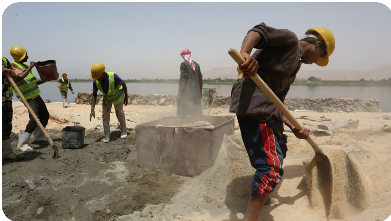
A project in Luxor, Egypt, creating short-term employment opportunities for unskilled and semi-skilled workers and providing access to basic infrastructure services. Photo: Dominic Chavez/World Bank
