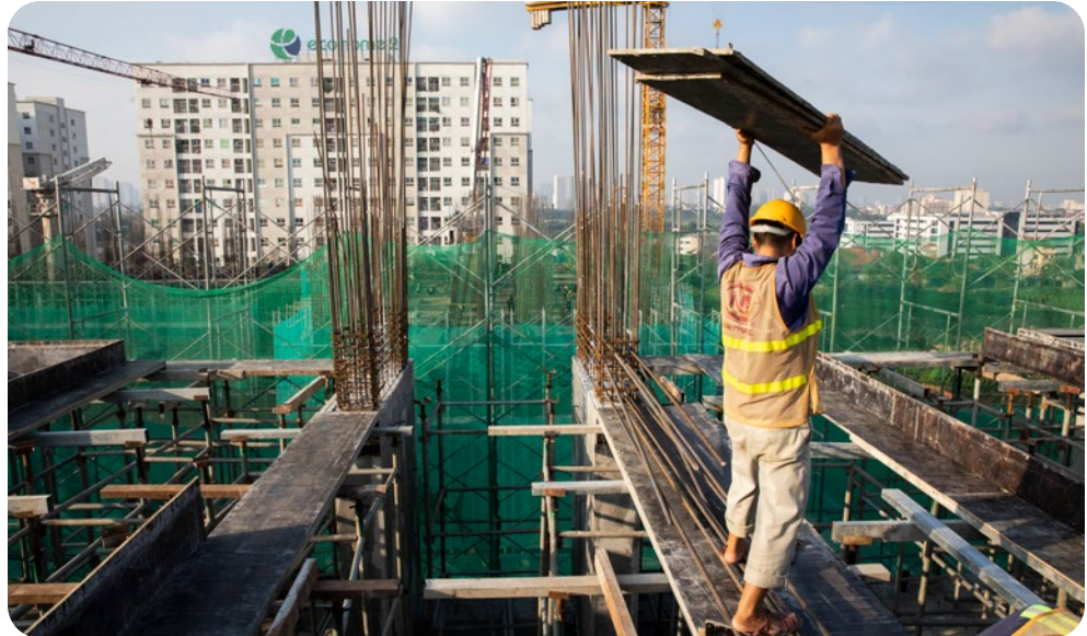
Construction worker preparing to pour concrete on an upper floor of the EcoHome apartment complex in Hanoi, Viet Nam. The finished towers will be EDGE certified and provide 2,197 affordable green apartments. Photo: © Dominic Chavez/IFC
