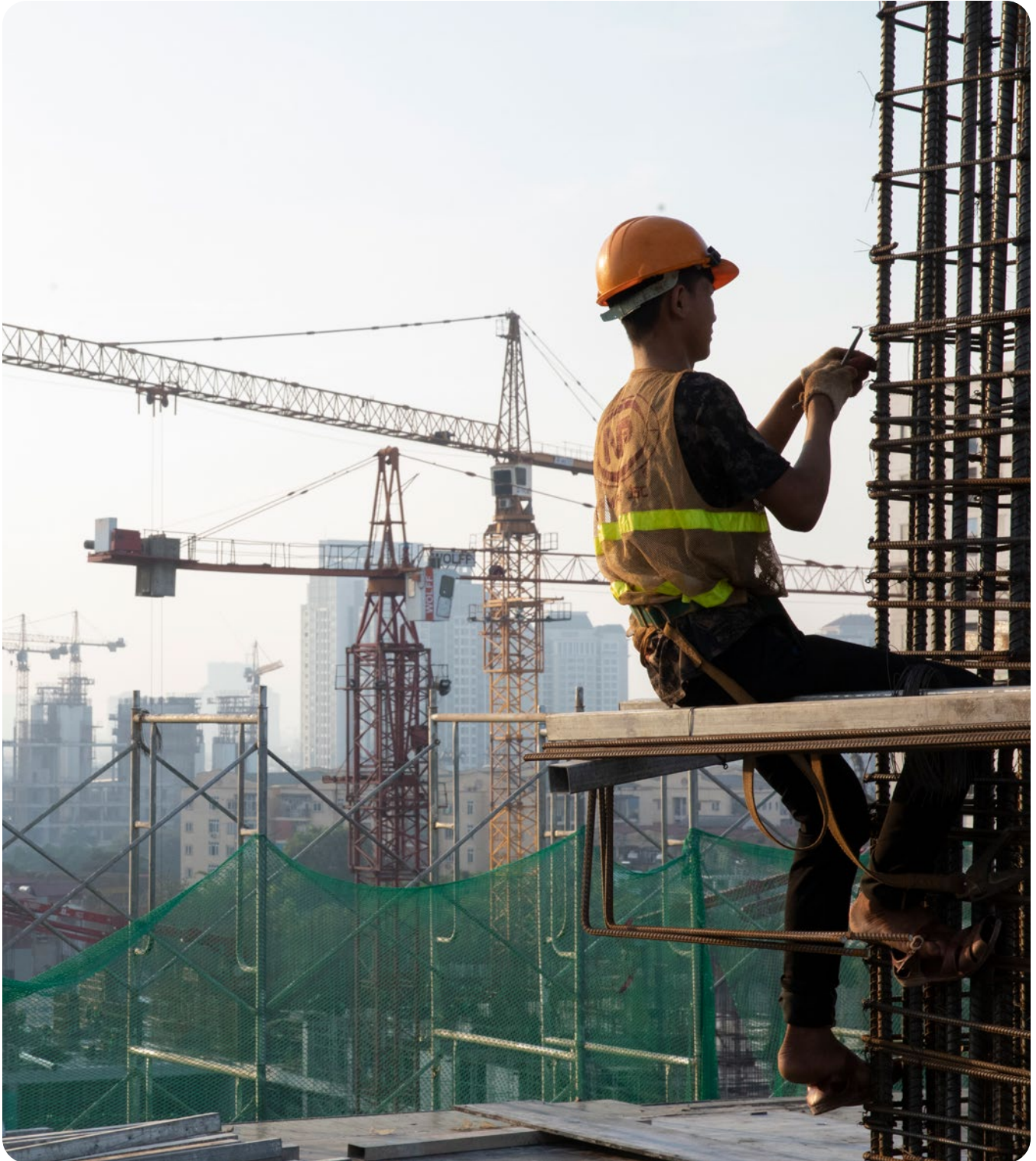
Construction worker preparing to pour concrete on an upper floor of the EcoHome apartment complex in Hanoi, Viet Nam. The finished towers will be EDGE certified and provide 2,197 affordable green apartments. Photo: © Dominic Chavez/IFC
